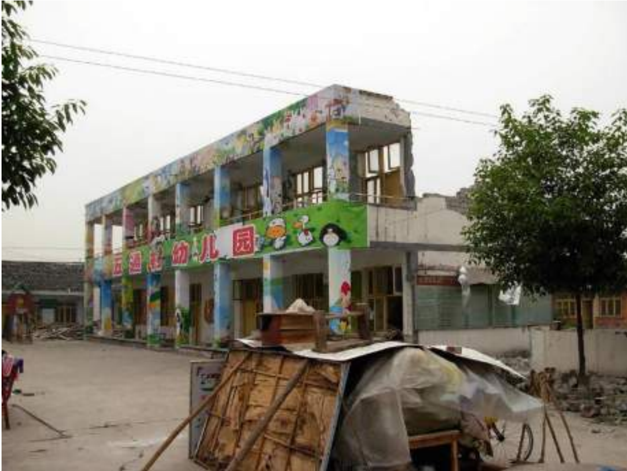
Fig. 8.3 This kindergarten was one of the many schools badly damaged, 2008 Sichuan earthquake. (Courtesy of Wikimedia Commons)
